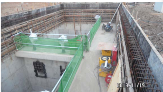
<Installations of electric flood gate>
