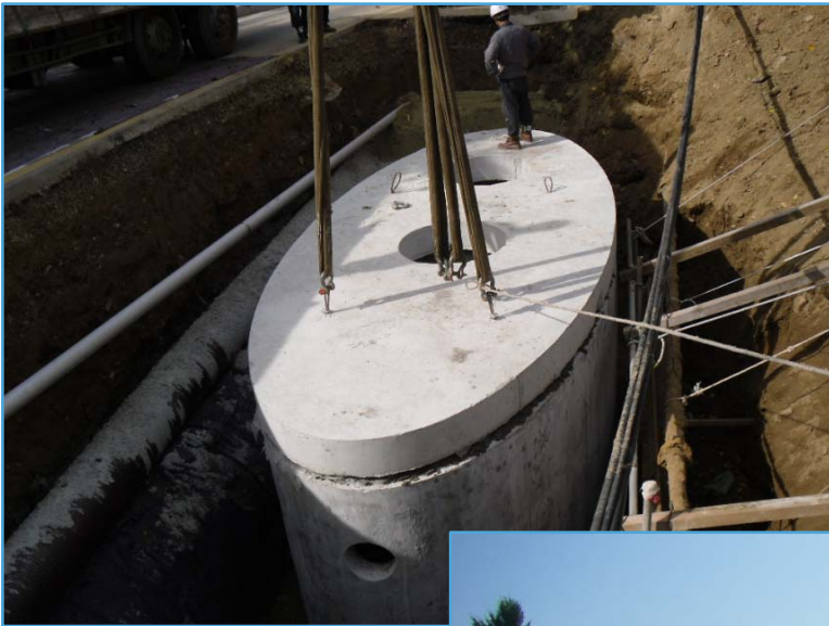
← <Installations of AOS SEPARATOR>
