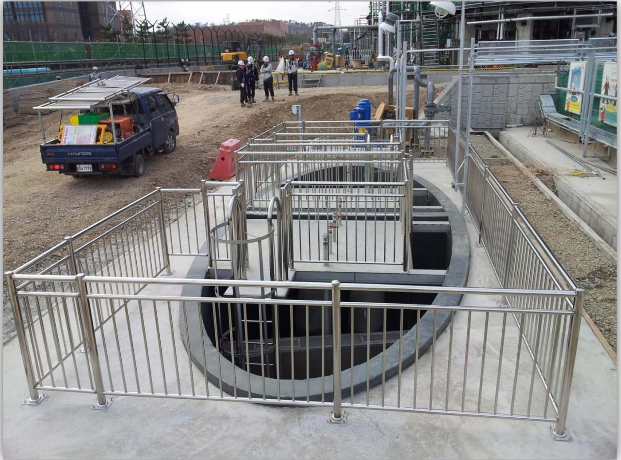
<Installations of AOS SEPARATOR>
