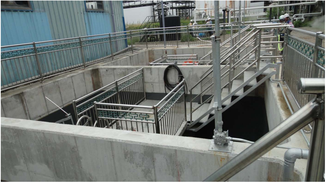
<Installations of AOS SEPARATOR>
