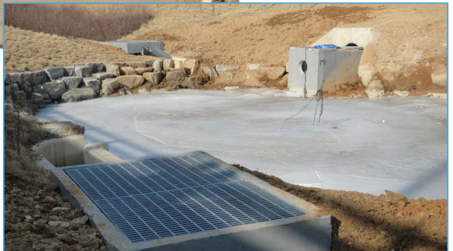
<collecting well type of non-point pollutants treatment equipment of vegetation water tank of Incheon Bridge >
