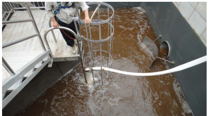
<Inflow of waste water before treatment>
