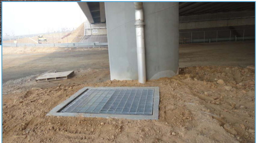
<collecting well type of non-point pollutants treatment equipment of drainage of Incheon Bridge>
